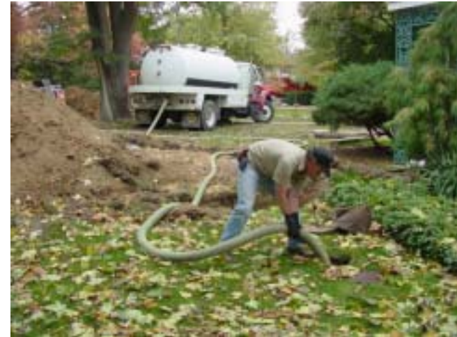
A septage hauler pumps a tank. Image courtesy of Roger Darr.
